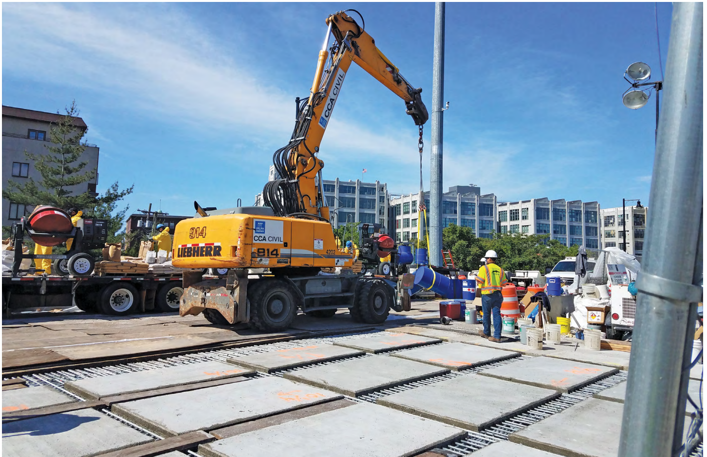
The Pulaski Skyway is a three-and-a-half mile, four-lane roadway in the northeastern part of New Jersey. The repair project on the eastern portion involved full demolition and replacement of the deck and repair of some of the structural steel.
